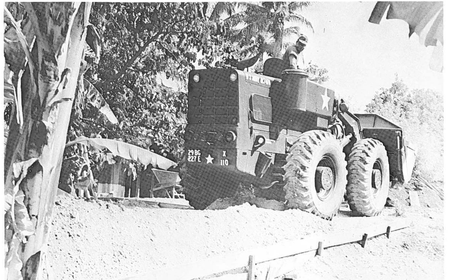
Ed Clark and his front loader graded a half-mile of pathway through the exhibit area.
