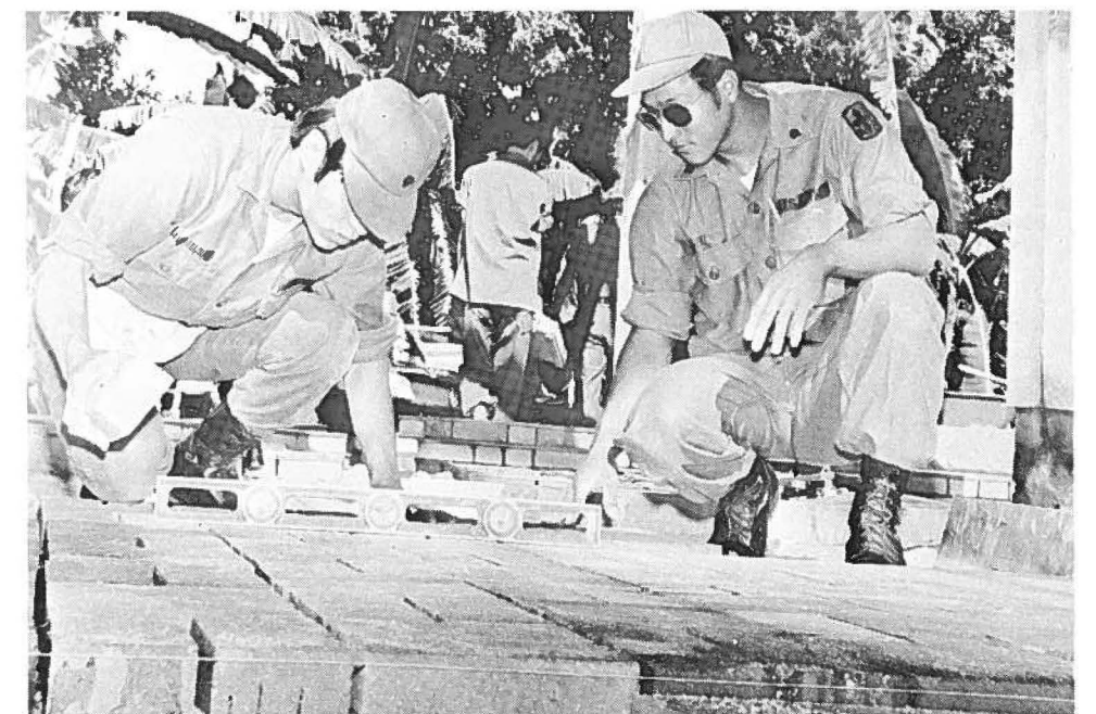
Other engineers laid the brick flooring for the market place area and exhibit pavilions.
