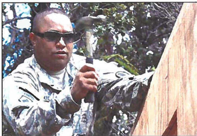
HAMMER TIME – Spc. Andrew P. Kalaukoa (right), a carpenter from Makaha, builds the outhouse roof.
