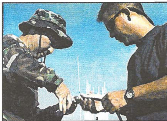
Tech. Sgt. Jimmy Kuwahara and Master Sgt. James Patao crimp a coaxial cable for a UHF antennae in a deployed location in support of Operation ENDURING FREEDOM.
