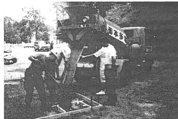
SET IN STONE - Spc. Nicole Y. Nishijo and Sgt. Arthur F. Sagon, 298th Engineer Detachment masons, along with civilian Japanese cement workers, pour the foundation for the pavilion being built at Camp Zama, Japan. Capt. Neal S. Mitsuyoshi photo
