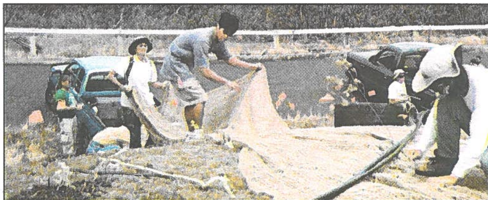
TEAMWORK — A bolt of Geojute is unrolled over the dusty bank of Diamond Head's Battery Harlow by Lincoln Yamashita, Shirley Zhai, Melissa Dumarán, Brad Uyeda, Paul Lyden, Melissa Ito, and Jennifer VandeBrake.
