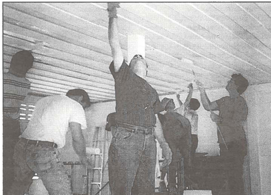
Hawaii Air National Guard's 154th Engineer Squadron repairs a school in Cambodia's capital, Phnom Penh, in April. (HIANG photo)
