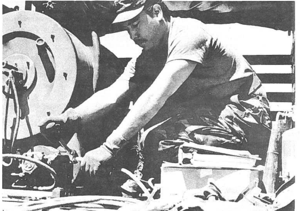
SAFE ADJUSTMENTS —Spec. 4 Patrick San Nicolas, 292nd Supply and Service Company, HARNG, uses gloves to adjust the water heater fuel-line for laundry support activities at George Air Force Base, California.
