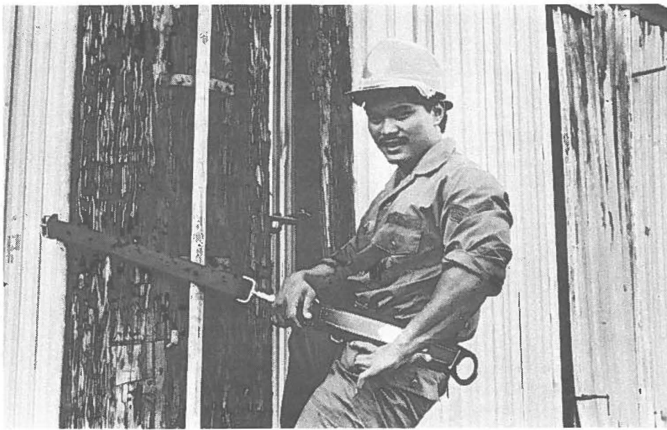
A "CHAMPION" HANG(S) FROM ABOVE—Senior Airman Dennis Cortez, 150th Aircraft Control and Warning Squadron, performs repair and replacement maintenance on radio antennas mounted on 90 foot poles when he is not training for body building competitions. (HANG photo)
