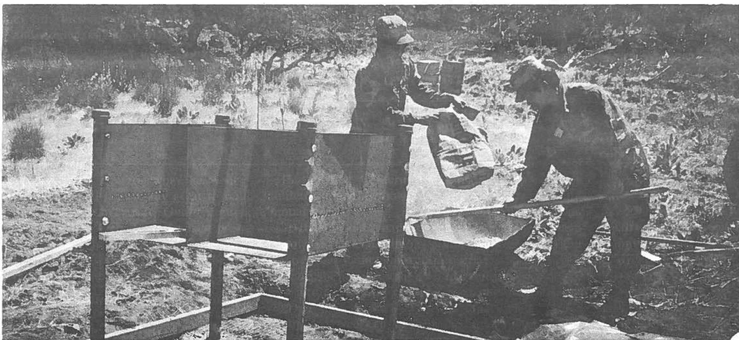
MAUNA KEA MIX—Spec.4 Lawrence Genobia (left) and Staff Sgt. Ray Asuncion, both from 198th Engineer Detachment, HARNG, mix concrete in preparation to build a barbecue broiler at the Mauna Kea
