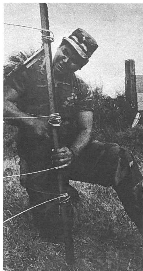
PULLING HARD—Sgt. Gregg Veal, 227th Engineer Company, HARNG, pulls a segment of wire fence taut at Kalapapa, Molokai. Photo by Staff Sgt. Dennis Fujii, 117th PAD, HARNG.
