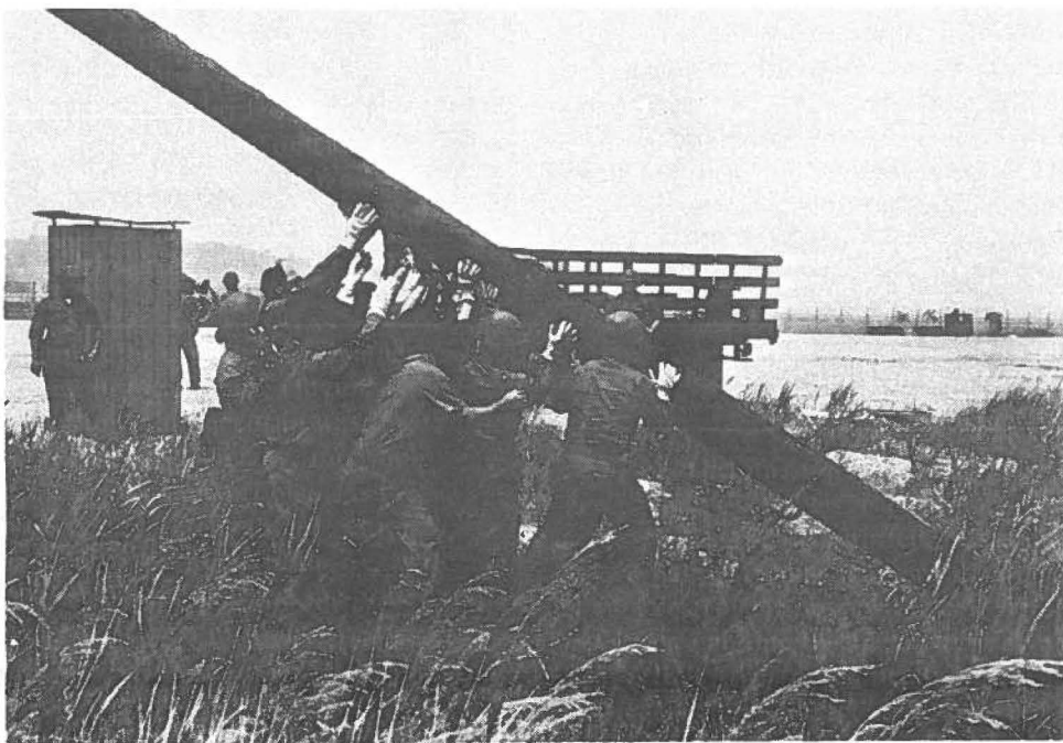
HOISTING THE POLES —Members of the 154th Civil Engineering Flight and the 432nd Civil Engineering Squadron electricians hoist the exterior lighting poles into place. Hawaii Air National Guard photo.
