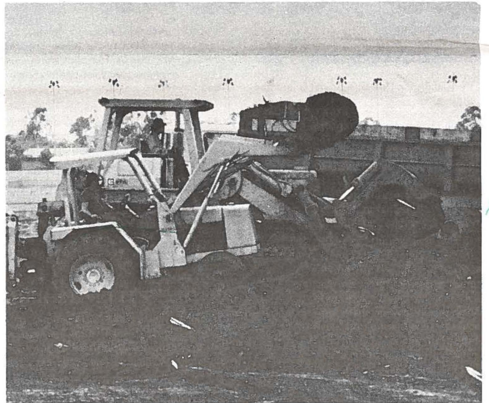
EARTHMOVING —Construction crews get to work on the new 300-man armory near the HARNG Aviation Facility, Wheeler Air Force Base.
