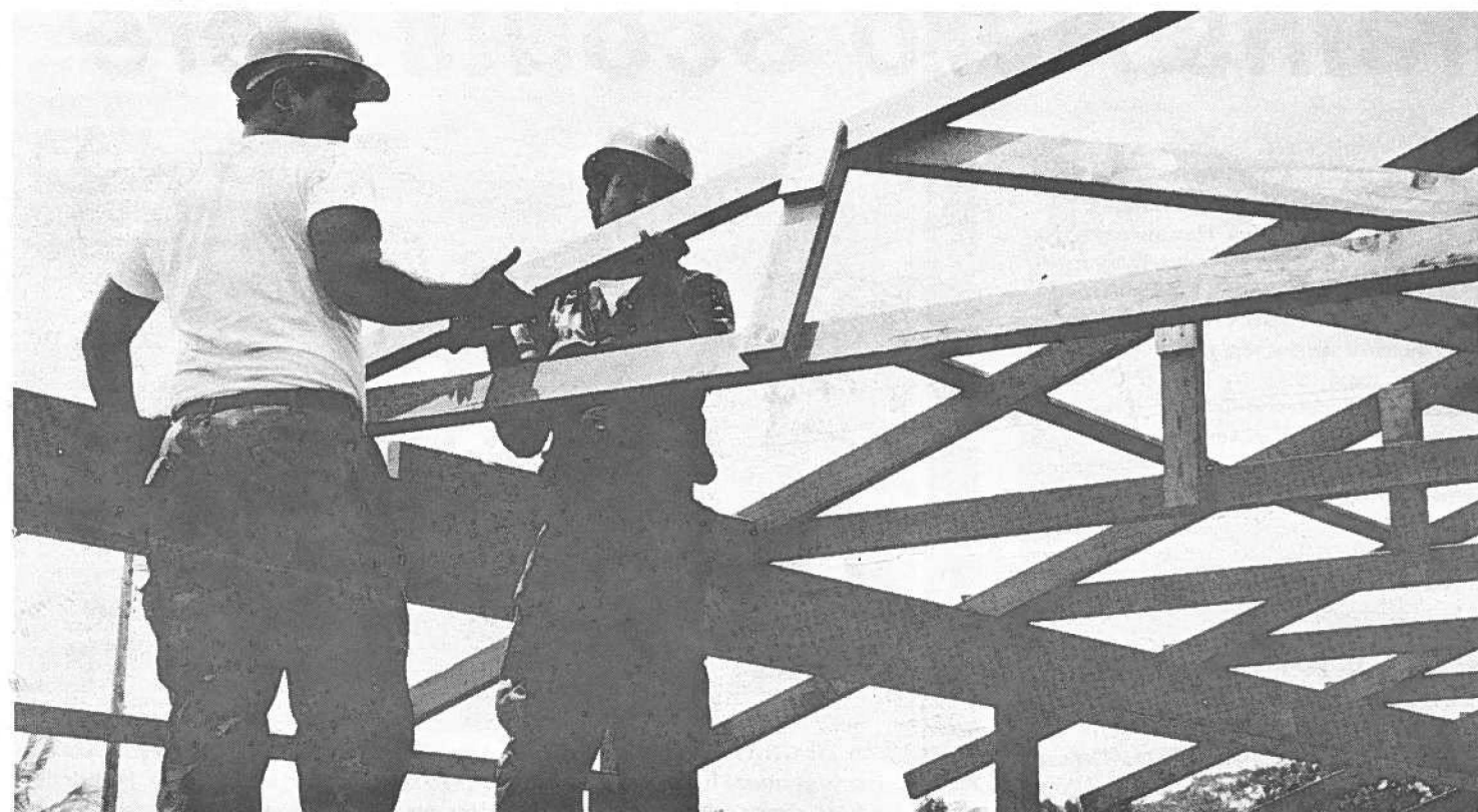
EASY DOES IT —Members of the 298th Engineer Detachment lift a roof frame on top a building at the Keaukaha Military Reservation during their two weeks of annual training. Hawaii Army National Guard photo by Capt. Bud Bowles
