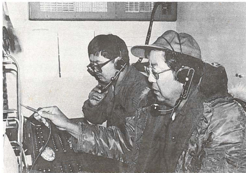
At the Sacheon switchboard, 201st members Staff Sgt. Allen Doi (left) and Sgt. James Takakura ensured that users were connected and calls completed.
