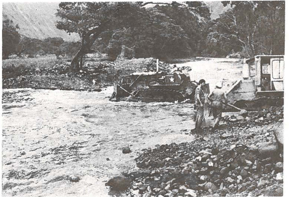
GUARDSMEN HELP CLEAN-UP AFTER BIG ISLAND FLOOD — Army National Guardsmen assist other State agencies during flooding caused by recent storms. Restoration was concentrated at Wailoa and Hiilawe streams in the Waipio Valley area.
