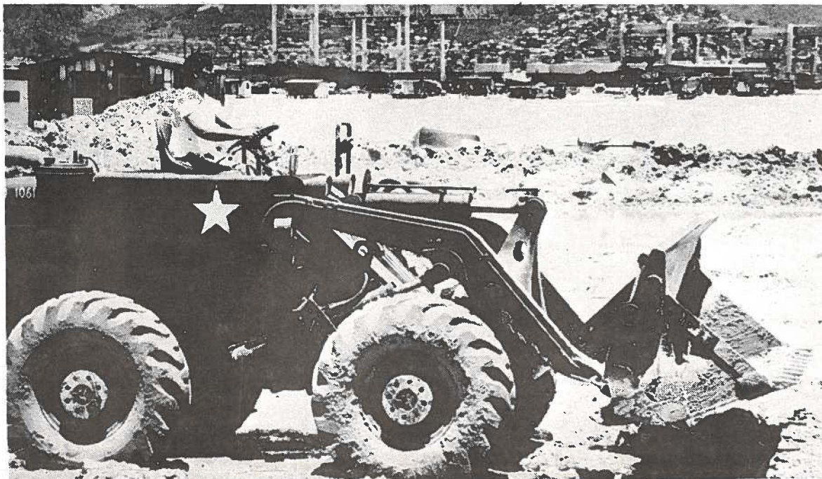
COMMUNITY SERVICE PROJECT — The Hawaii Army Guard's 298th Engineer Detachment assist in the restoration of Mokauea Island fishing village. 117th PAD photo by Sp4 Tom Clements.
