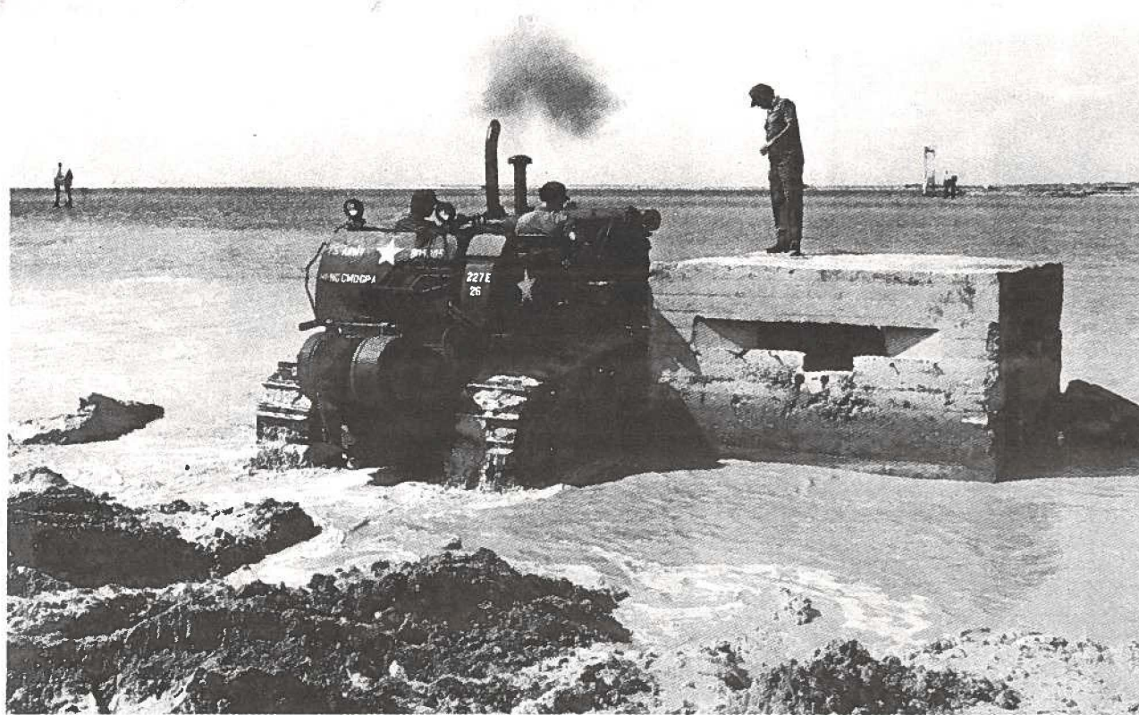
SEA GOING TRACTOR — Member of the 227th Engr. Co., aided by a bulldozer, scrape the sand surrounding a 18-ton bunker in efforts to move the bunker.
