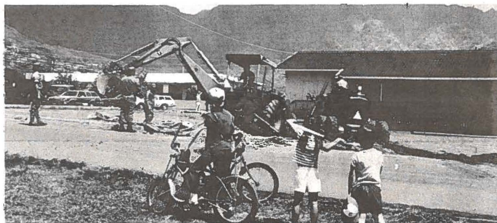
COMMUNITY SERVICE PROJECT — The Army Guard's 298th Engineer Detachment works on a road for Manoa Elementary School. The purpose of the community service project was to alleviate the hazard of cars cutting across the school. — Photo by Sp5 John Atkinson.
