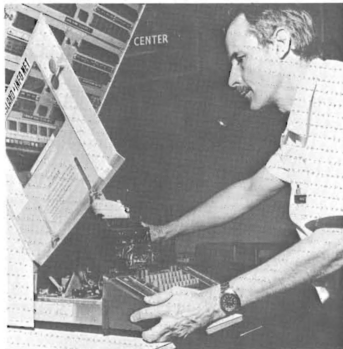
New radio and teletype equipment increased State CD communications capabilities during FY 71.
