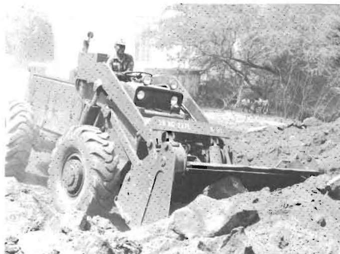
DIGGIN' IN —SP5 David Keamo, 227th Engineer Company heavy equipment operator, maneuvers his front end loader into a pile of dirt and rock adjacent to Ruger Theatre where the Engineers assisted Honolulu Community Theatre in clearing and grading land for construction of a new scenery and costume shop.
