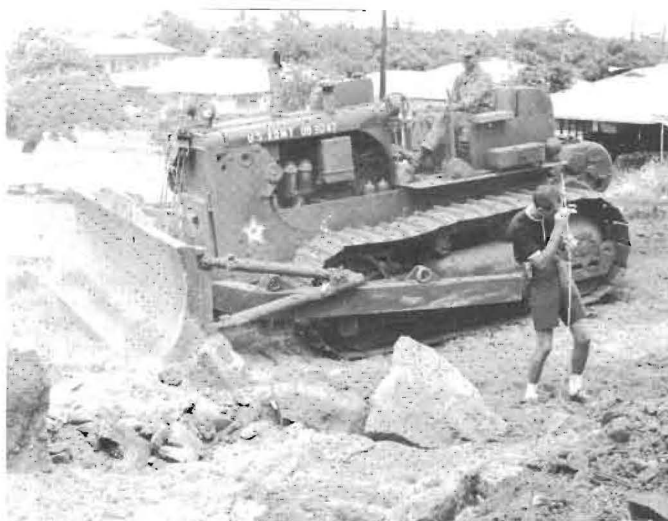
SURVEY —While SP5 Allan Hardy, 227th Engineer Company clears and grades the property adjacent to Ruger Theatre, Frank Herman, a volunteer worker for Honolulu Community Theatre checks the grade. The 29th Brigade's Engineers assisted HCT in preparing the ground for construction of a new scenery and costume building.
