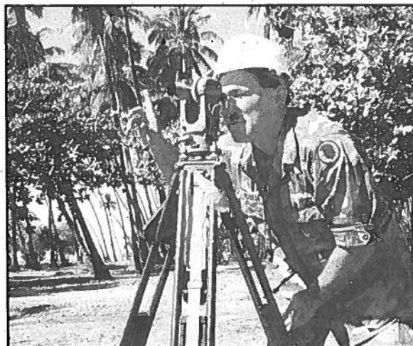
EVEN PLANE — Sgt. Vance L. Vidinha, 298th Engineer Detachment, directs the leveling of the area being prepared for the foundation of the new pavilion at Kalama'ulu Homestead's Ki'owea Beach Park, Molokai. 1st Lt. Jeffrey D. Hickman photo
