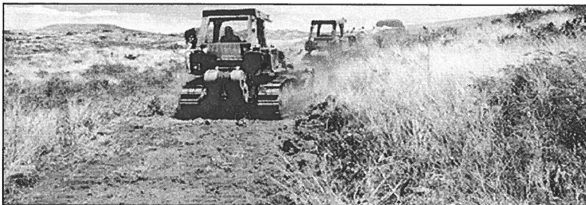
ON THE ROAD TO KAHIKINUI — Soldiers from the 298th Engineer Detachment cut Maui's Operation KAHIKINUI road. The operation built access roads for the Department of Land & Natural Resources' Hawaiian Homes homestead project. Spc. Vincent Maloney-Cui photo
