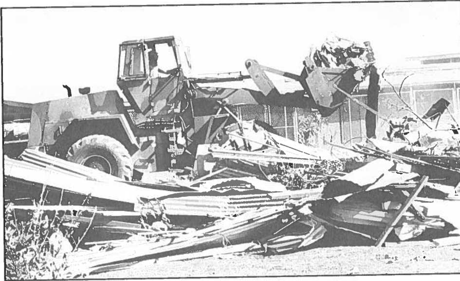
A heavy equipment operator from the Hawaii National Guard's 227th Engineer Company clears debris from Kapaa High and Intermediate School using a scoop loader.
