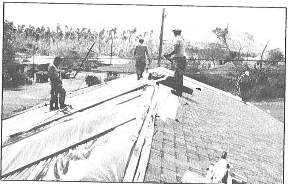
Soldiers from the Hawaii National Guard's 298th Engineer Detachment repair the roof for a Kapaa, Kauai family whose father was recovering from a stroke, September 1992.
