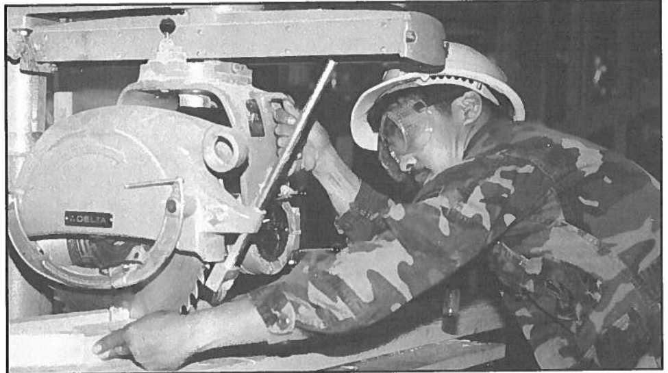
An airman from the 154th Civil Engineering Squadron cuts wood for a minor construction project at Kulis Air National Guard Base, Alaska, in July.
