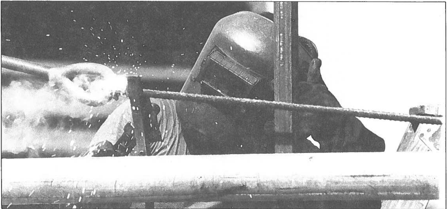
A 227th Engineer Company soldier welds a cable to the Kaena Point wild life refuge gate built to restrict access of motorized vehicles. The environmental enhancement project is Federal funded yearly.
