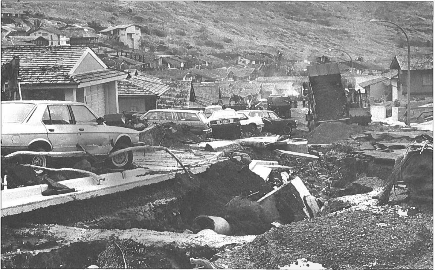
In the aftermath of Oahu's New Year flood, Hawaii Army National Guard dump trucks from the 227th Engineer Company brought in loads of dirt and gravel to repair the eroded Kahena Street. The temporary by-pass on Kahena Street enabled cars to be removed following the worst flood in Oahu's history.
