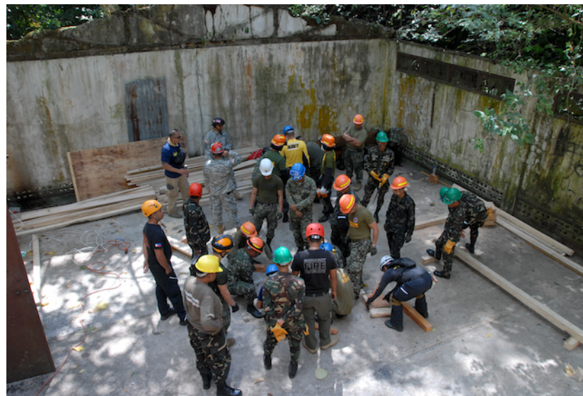
Members of the Philippine Armed Forces practice Spot "T" shoring. Shoring rein enforces a collapsed structure making it safer for first responders to enter. Camp Lapu-Lapu, Cebu, Philippines, Mar. 3, 2014. (U.S. Air Force Photo/SrA Orlando Corpuz)
