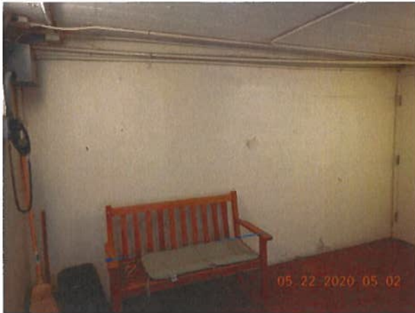
Photo 37 – Lead Dust Hazard W-07
