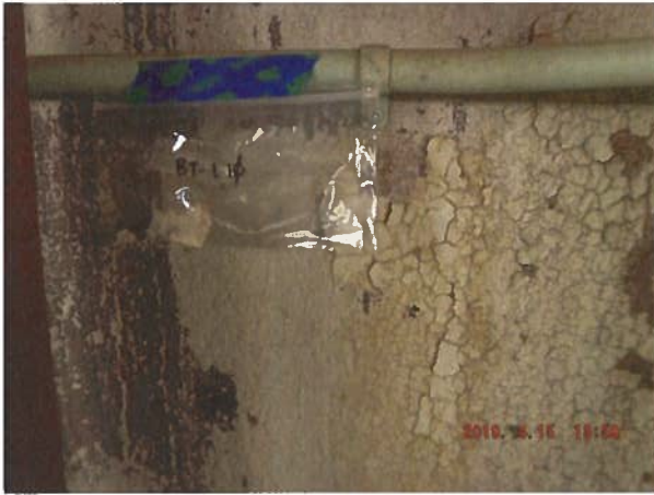
Photo 19 – LCP L-10 (close-up)
