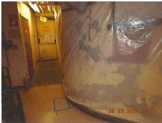
Photo 41 – Lead Dust Hazard W-15
