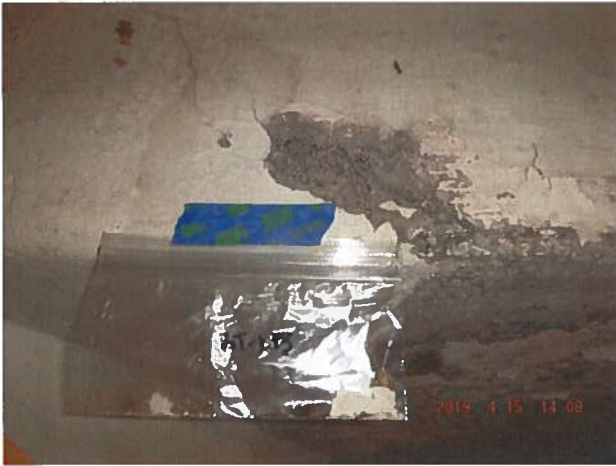
Photo 25 – LCP L-13 (close-up)
