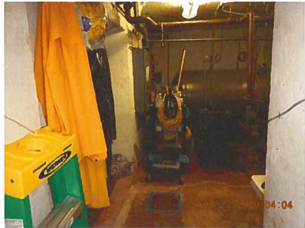
Photo 40 – Lead Dust Hazard W-13
