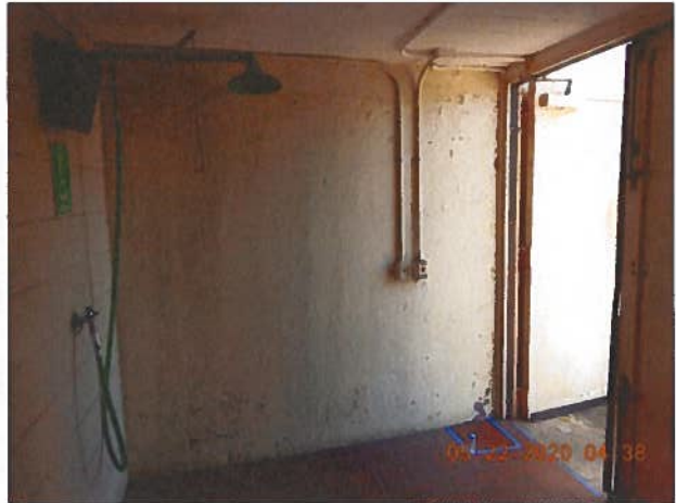
Photo 38 – Lead Dust Hazard W-08
