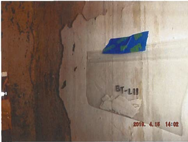
Photo 21 – LCP L-11 (close-up)
