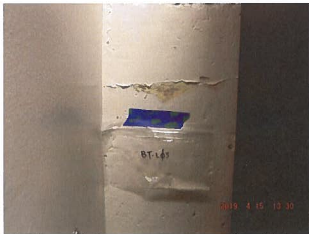
Photo 5 – LCP L-03 (close-up)
