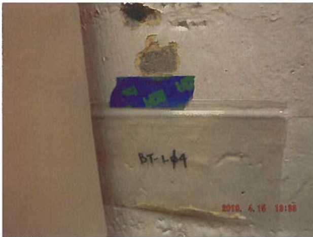
Photo 7 – LCP L-04 (close-up)
