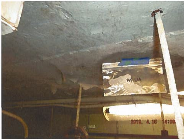
Photo 27 – LCP L-14 (close-up)
