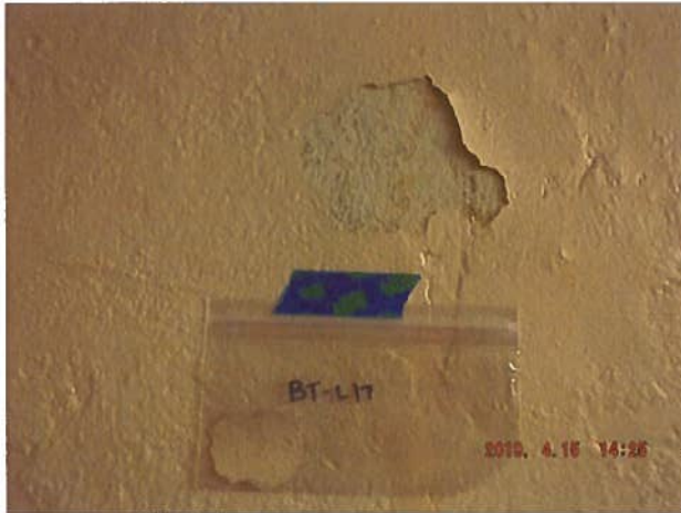
Photo 33 – LCP L-17 (close-up)
