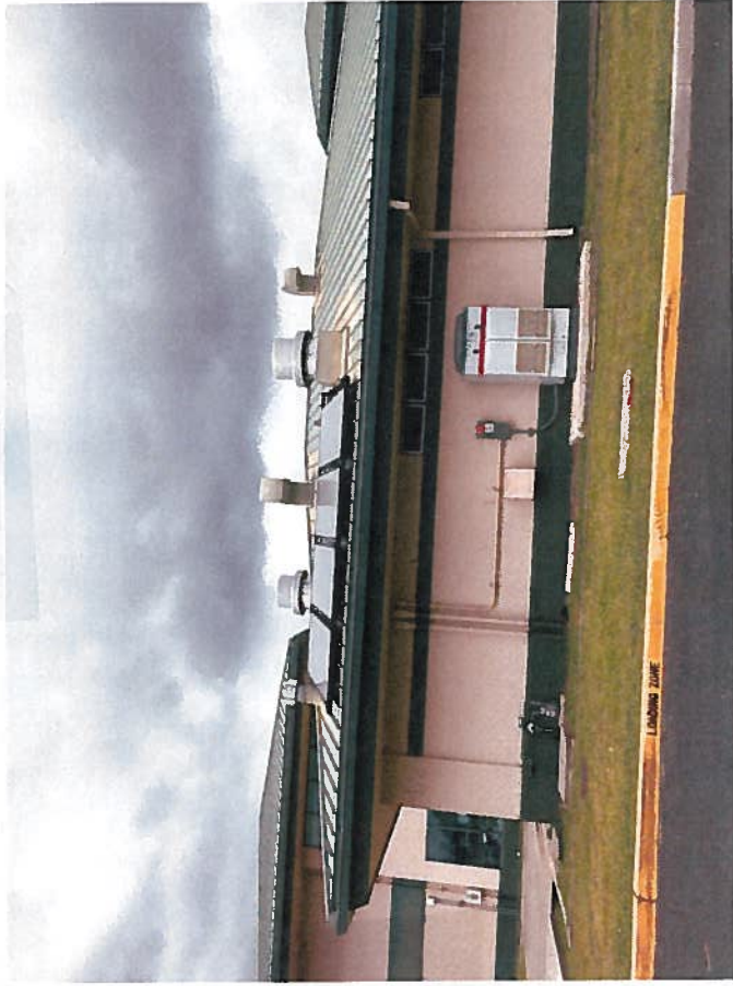
PV Panels location on roof side 2
