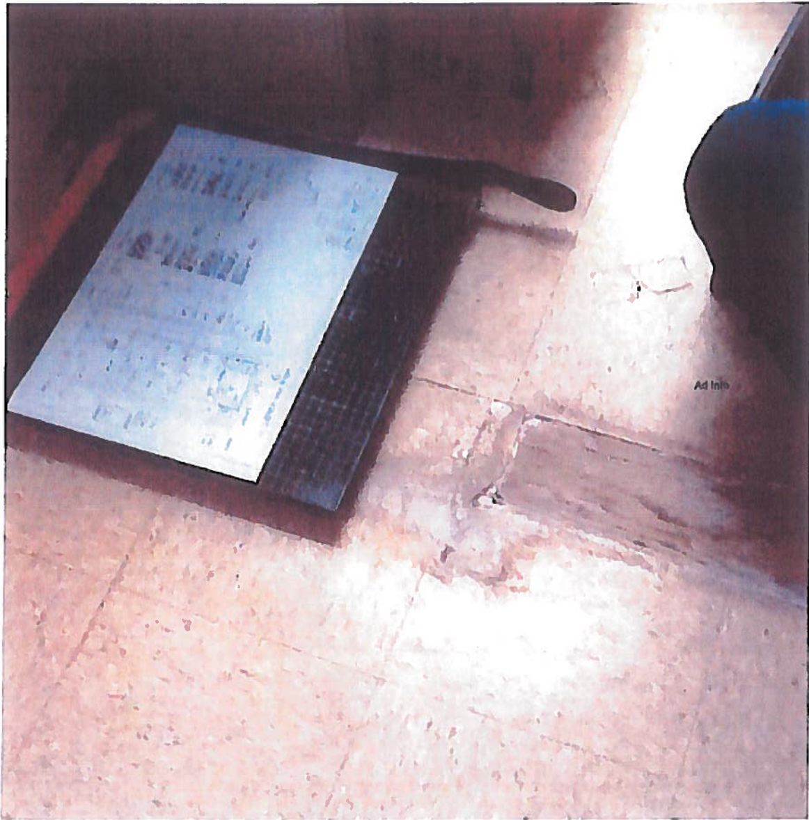
BUILDING 306 ALPHA - ROOM 228
