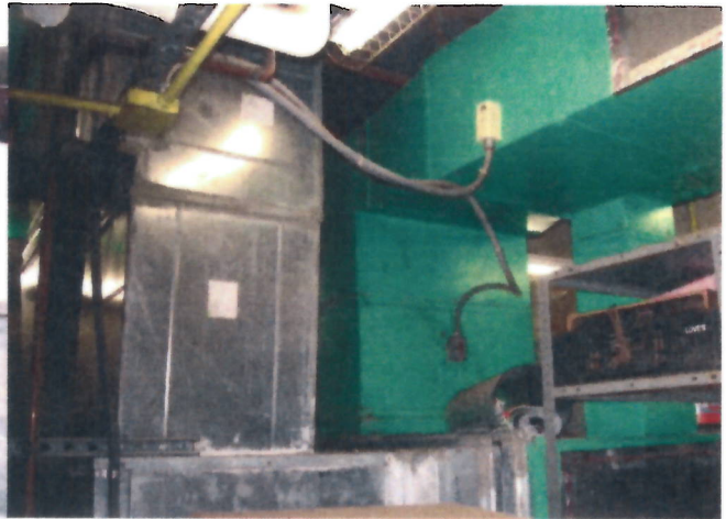
Photograph 2 View ventilation and air-conditioning unit in the mechanical room
