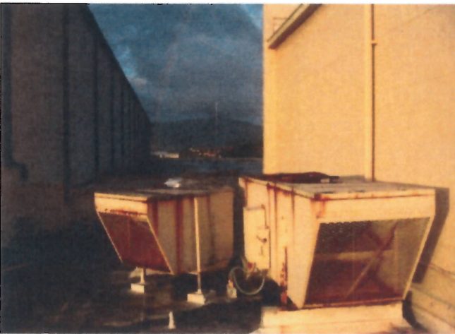
Photograph 3 View of make-up air units for the kitchen
