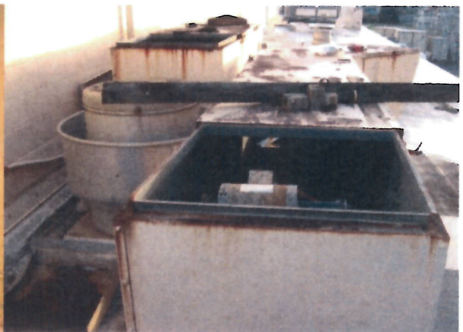
Photograph 4 View of make-up air units for the kitchen
