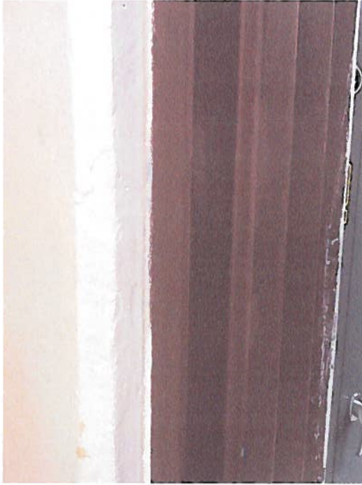
Sample Area # 302-46-1W white caulking at door frame
