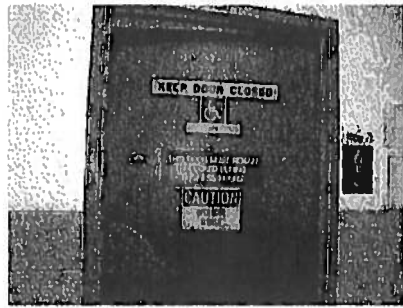
Photo #32 Building 308A 1st floor, men's bathroom, lead-containing brown lower CMU wall and non-lead containing white upper CMU wall.
