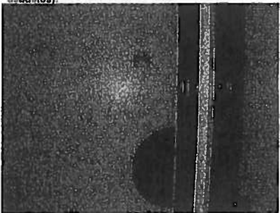
Photo #6 Building 306, 1st floor men's restroom, lead-based brown metal door frame and lead containing white wood door.
