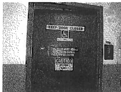
Photo #30 Building 306A, 1st floor, men's bathroom, lead-based gray metal door frame.
