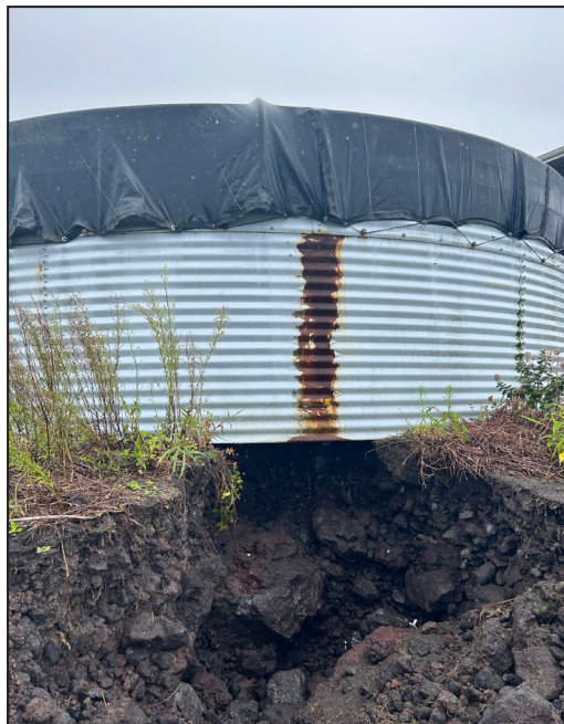
Damage to tanks disrupted a critical life-line for residents who rely on catchment systems for their water supply. Photo: HIEMA
