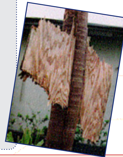
Cover photo: The roof and upper floor of this home received major wind damage from Hurricane Iniki in September 1992 (Photo: FEMA) Below: Plywood spears a palm tree during hurricane Andrew in August 1992.
