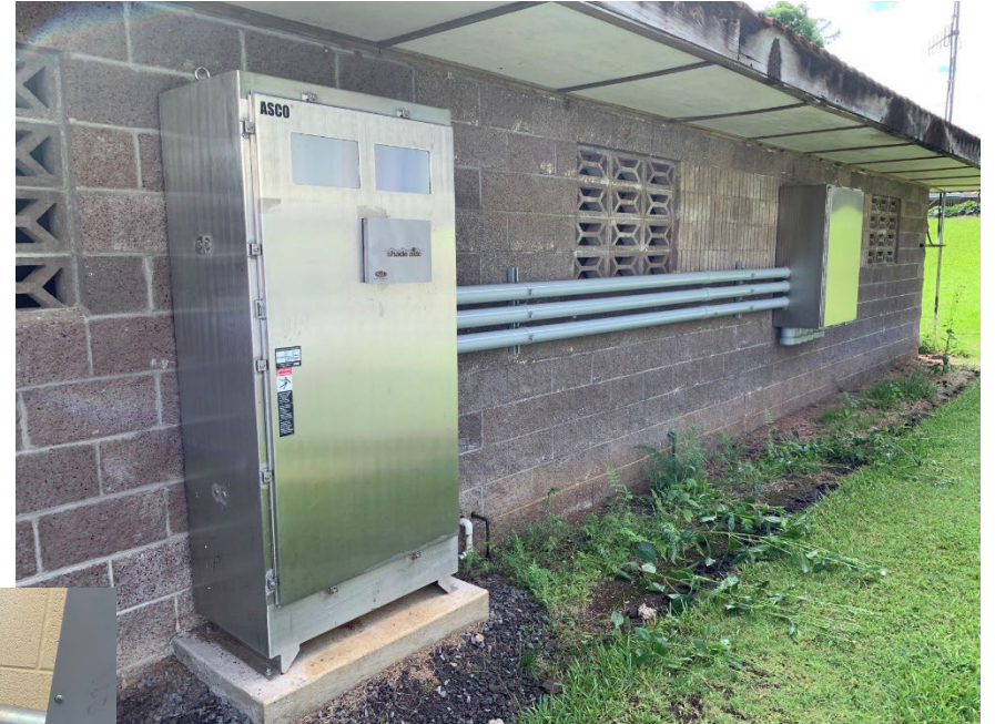
Piihonua – Transfer Switch and Term Box
