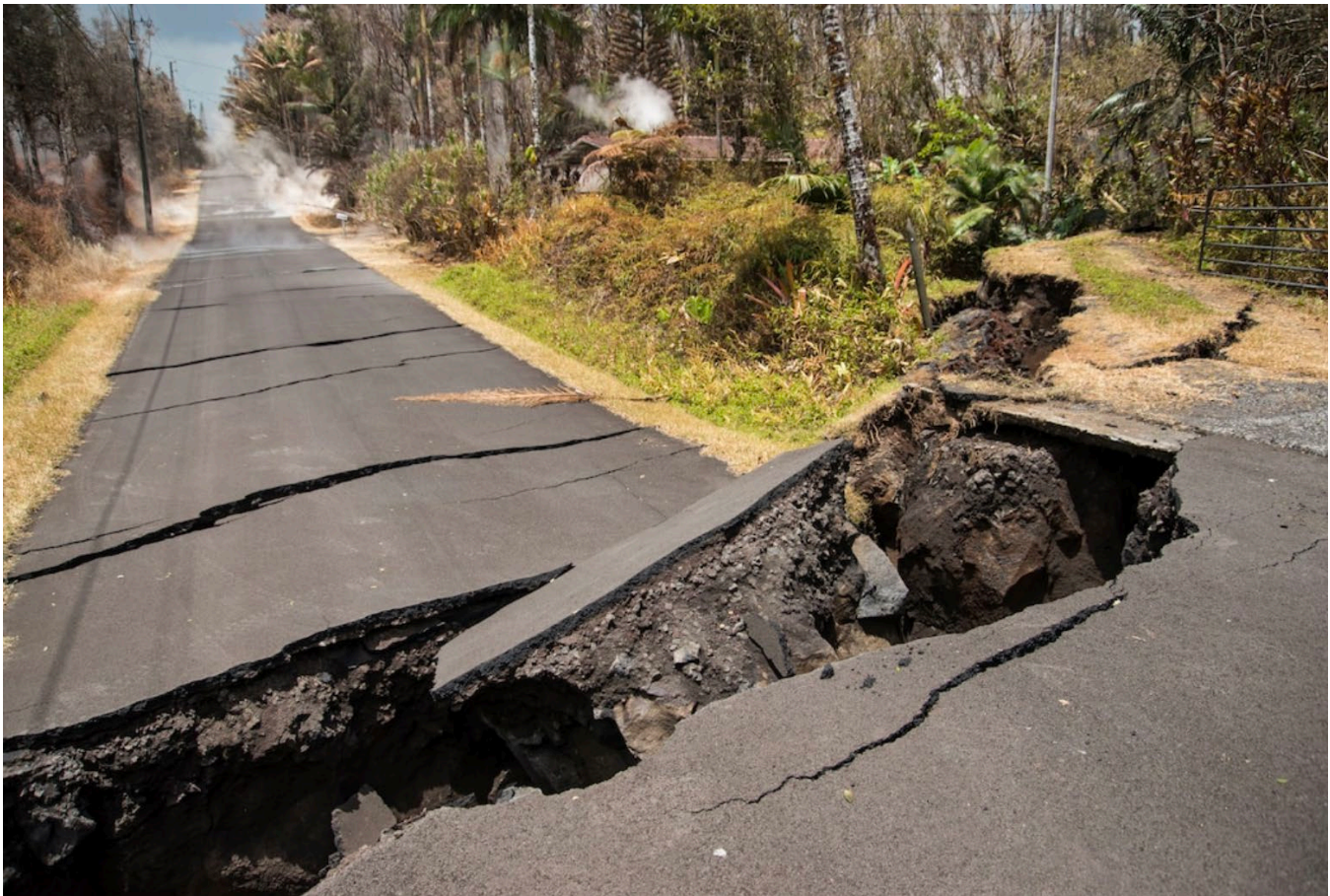
Figure 4.5-1. Road Damage from a Tectonic Earthquake in Hawai’i County, 2018
