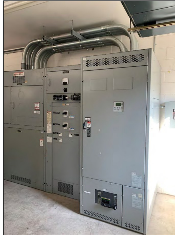
Honokōhau Transfer Switch
