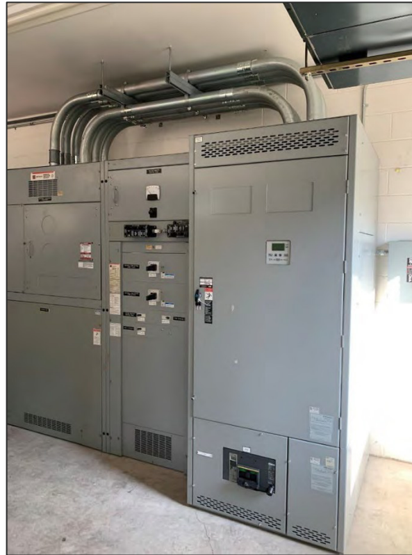
Honokōhau Transfer Switch
