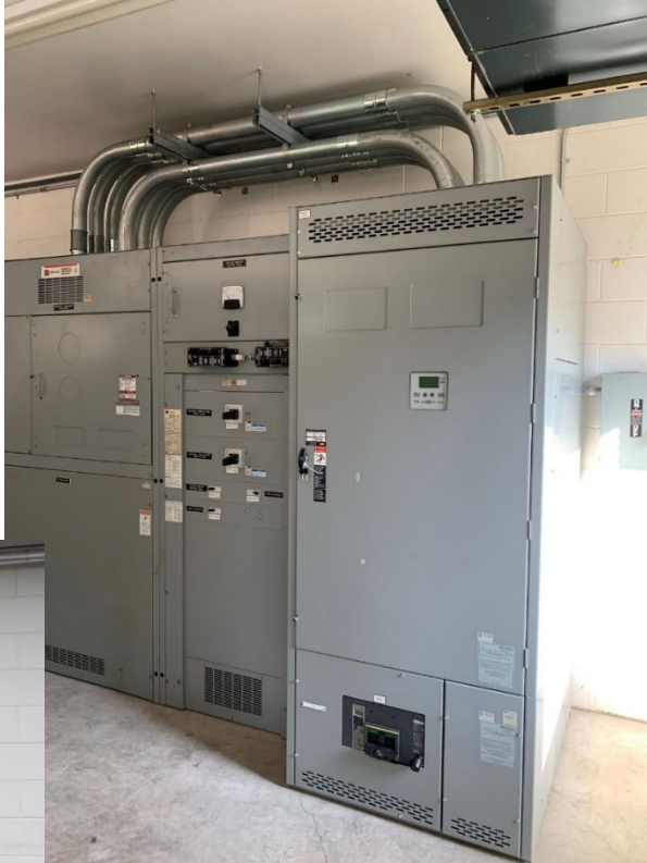
Honokohau – Transfer Switch
