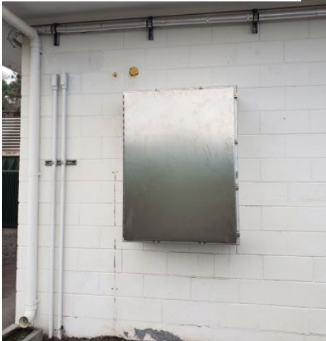
Honokohau – Termination Box
