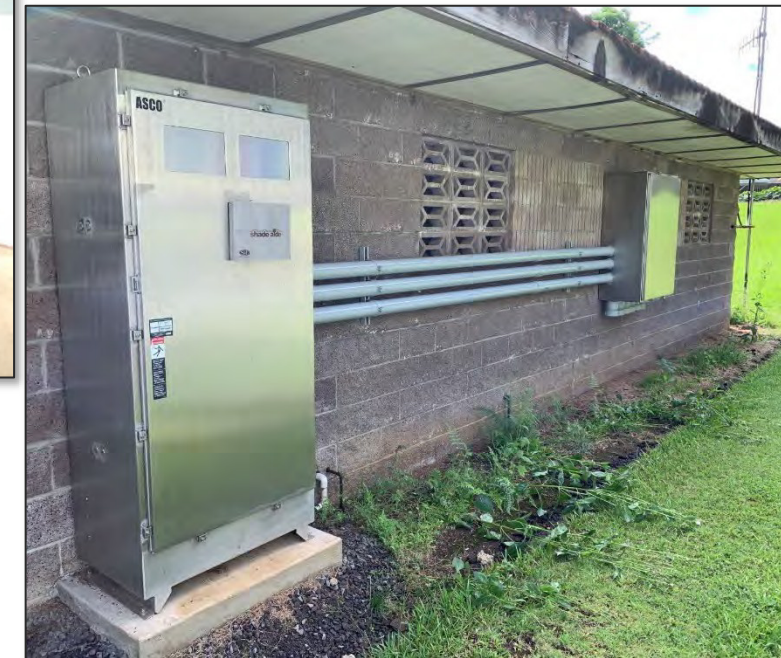
Pi'ihonua Transfer Switch and Terminal Box
