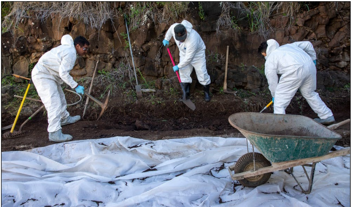
Figure 4.7-3. Naval Employees Relocate Soil Contaminated by Aqueous Film Forming Foam (AFFF) Concentrate in 2022
