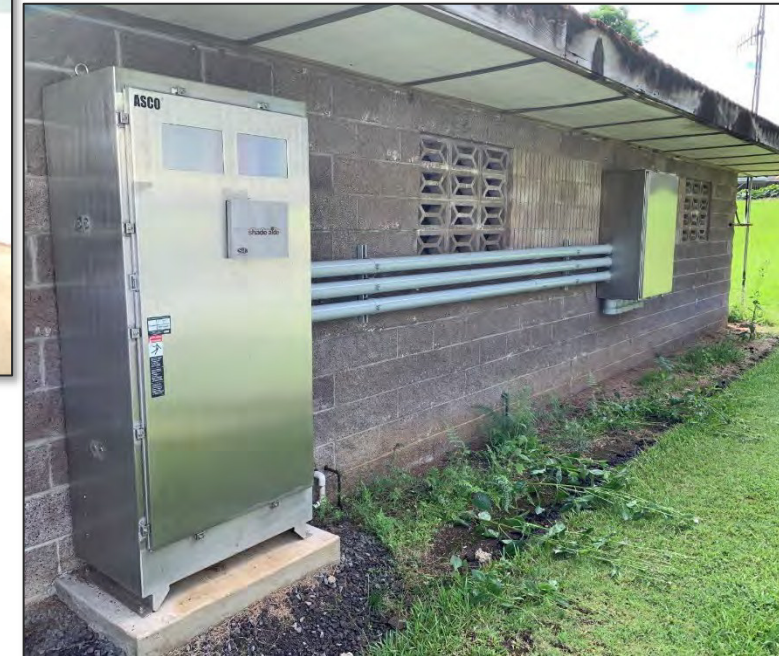
Pi'ihonua Transfer Switch and Terminal Box
