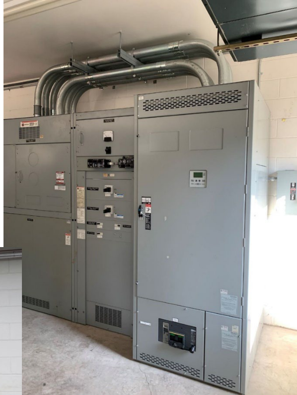
Honokohau – Transfer Switch
