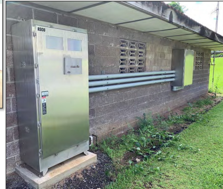
Pi'ihonua Transfer Switch and Terminal Box
