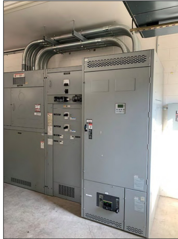
Honokōhau Transfer Switch
