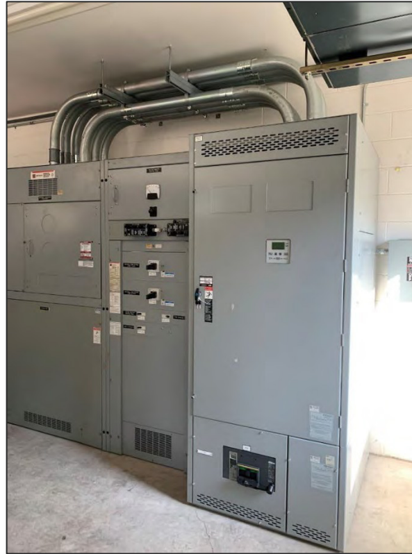
Honokōhau Transfer Switch
