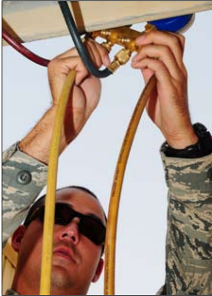
Staff Sgt. Brandon Ozaki, 386 ECES Heating, Ventilating, and Air Conditioning journeyman, recovers refrigerant from a packaged air conditioning unit at an undisclosed location in Southwest Asia Aug. 5. (U.S. Air Force photo/Tech Sgt. Tony Tolley)
