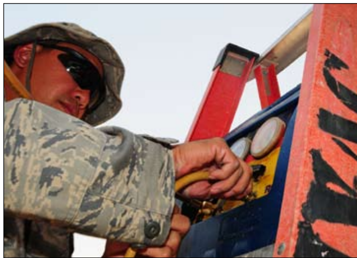
Airman Christopher Aurio, 386th Expeditionary Civil Engineer Squadron Heating, Ventilating, and Air Conditioning apprentice, prepares to recover refrigerant from a packaged air conditioning unit at an undisclosed location in Southwest Asia Aug. 5. Airman Aurio is deployed from the 154th Wing, Hickam Air Force Base, Hawaii. (U.S. Air Force photo/Tech Sgt. Tony Tolley)
