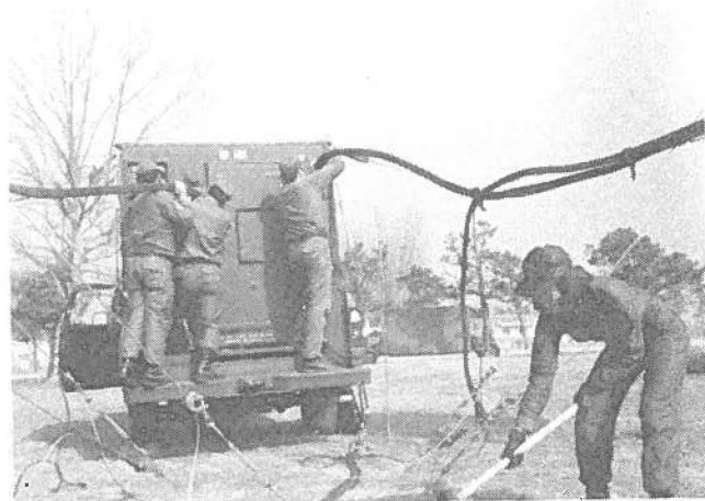
SrA Cody S. Nakasone, 202 CMBTCF, HANG, hammers antenna tie-down stakes during the installation of the communications operations at Suwon. Team Spirit '79.
