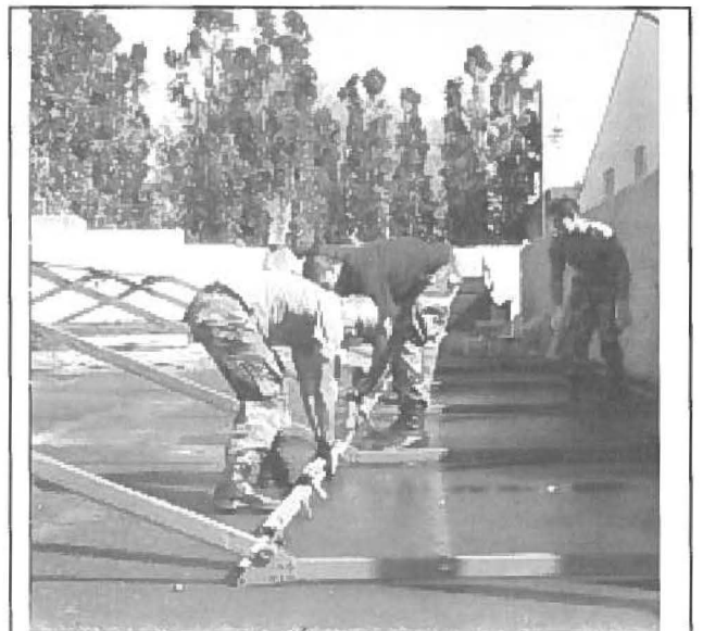
154 SVF members assembling a temper tent prior to moving to their deployed site at zone F.
