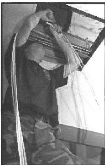
Member of the 154 CF deployed to Pease AFB to help in the installation of network and other cabling. Photo by SSgt Kristen Higgins, 154CF/SCV
